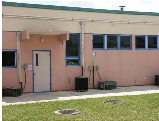
Figure 7. Blue tape used to seal doors and windows in fumigated structures with impermeable exterior walls in Florida. Walls in the Azores are also of impermeable composite covered with stucco (from Scheffrahn et al., 2006).
