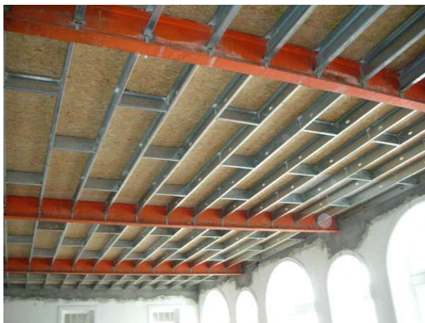
Figure 3. Renovation of the Catholic seminary with metal frames, after original building was damaged by C. brevis .
